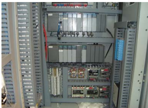
Panel de Control Waukesha PTA Pichanal (TGN SA)
